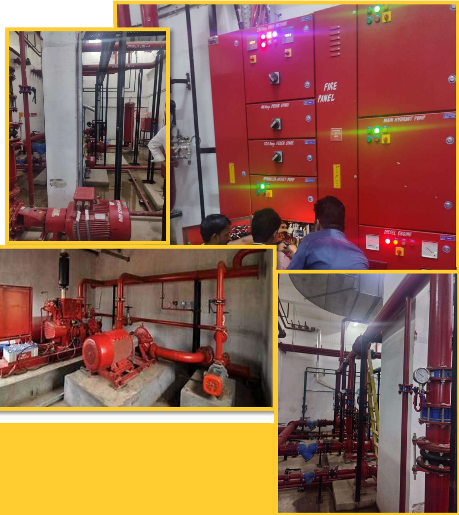
* Execution of Fire Pump Room and Fire Alarm Control Panel Room works at Yotta Data Centre, Greater Noida *
